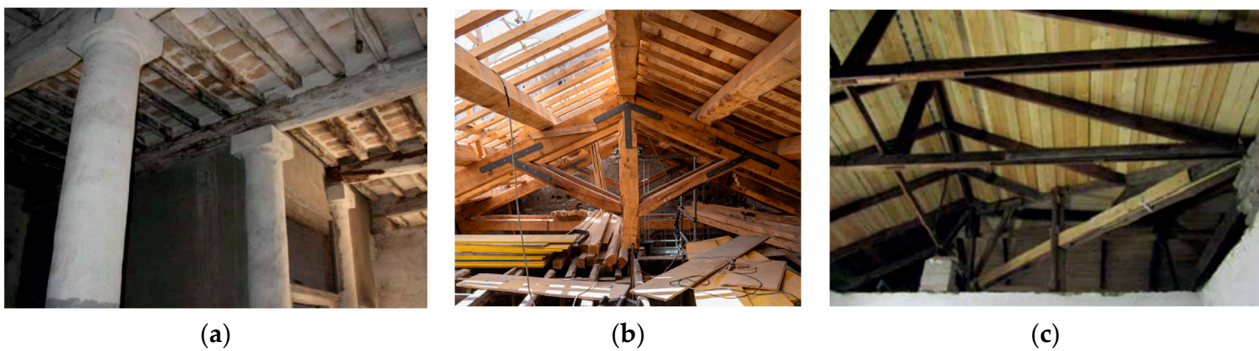
Figure 5. (a) Scuderie della Rocca Benedettina di Sant'Apollinare in Perugia: replacement of the damaged wooden elements; (b) San Giuseppe dei Falegnami: new wooden roof after the collapse in 2018; (c) Palazzo Silvestri-Rivaldi: coating with external photovoltaic elements.
