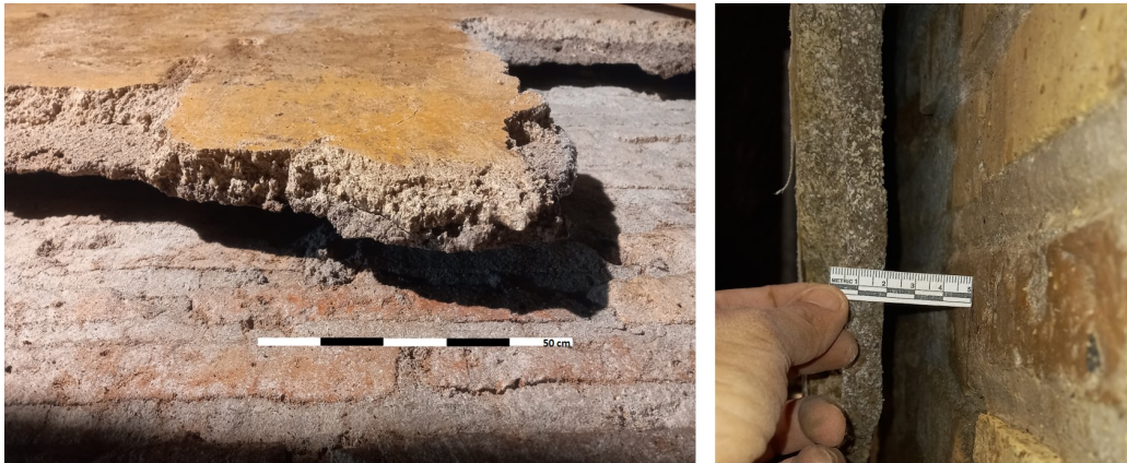
Figure 2: Detached plaster on the south wall
