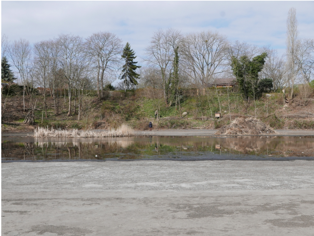
Plate 2. View of the slope forming the detention basin. The photo depicts a moment of vegetation maintenance, in particular the pruning of trees. Photo credits: Federico Brogini.
