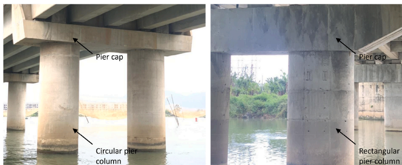
Fig. 2. An example of typical RC simply supported bridges with rectangular and circular cross-section columns in Da Nang.
