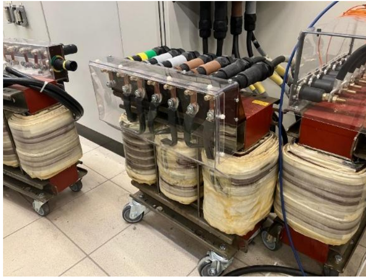
Figure 76: Additional inductance in series to the EGSTON-side transformer.
