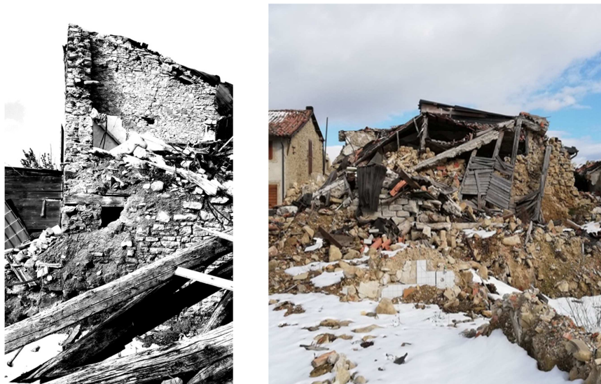
Figure 1. Damage scenarios after the Central Italy earthquake sequence (2016-2017) in the municipality of Accumoli (Rieti).
