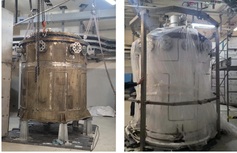
Figure 2.14: On the left, a picture of the stainless steel tank installed. On the right, the SST after the insulation with 20 cm thick Polyurethane.
