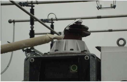
Fig. 1. Collapse of a HV circuit breaker from the Emilia-Romagna earthquake (Italy).
