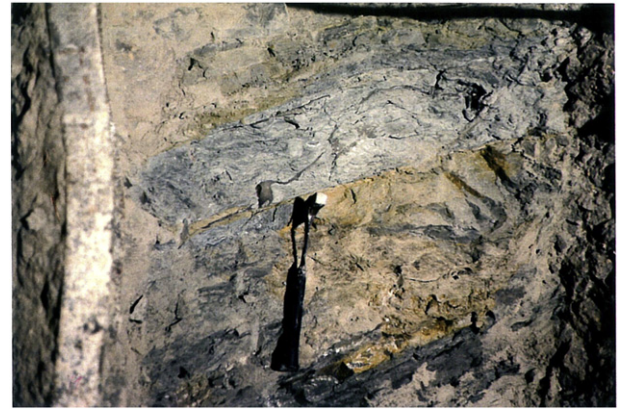
Fig. 8. Clay gouge interbed exposed in the damaged tunnel section; the thickness of the clay layer is approximately 0.2 m; on the left, a deformed steel set is visible.
