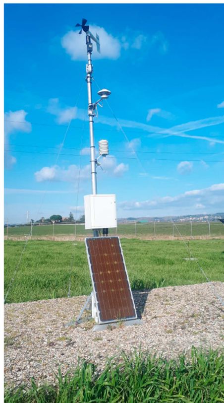
Figure 4. SMART metering system of PV plant.
