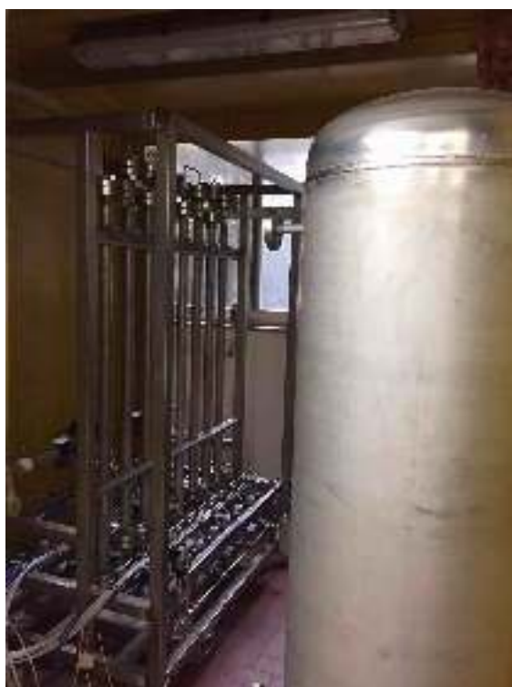
Fig. 5. Test plant used for characterizing and selecting sorbents for the UAr extraction plant PSA unit.
