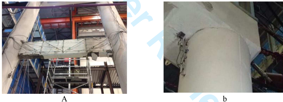
Figure 23. Damage state of Pier #11 after HS k12: a) transverse beam damage; b) crack opening underneath the cap beam.
