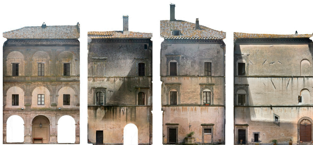
Figure 12. Orthophotos of the courtyard facades, obtained in Agisoft Metashape from the meshed and textured model. The quality of the mesh and texture allows, in many cases, detailed tracing of the entire ornamental apparatus and mapping of the deterioration of heavily damaged and incomplete materials (image by the authors).
